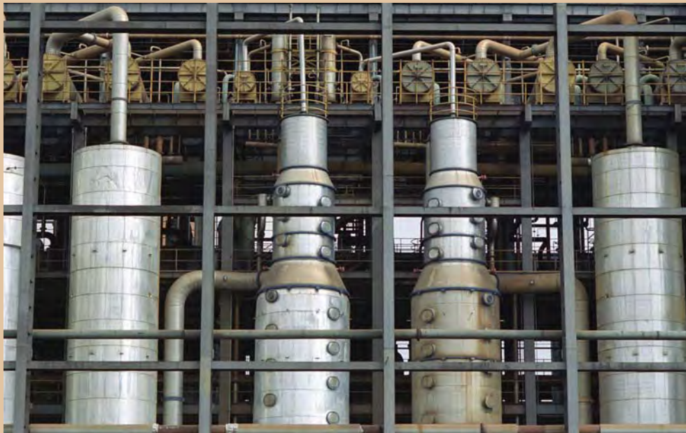
Brazil is the world's foremost producer of biofuels. Above, distillery in Brazil, for sugar and ethanol production.
